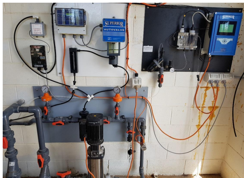
Chlorine trimming system
