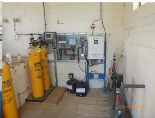
Chlorine Gas Room
