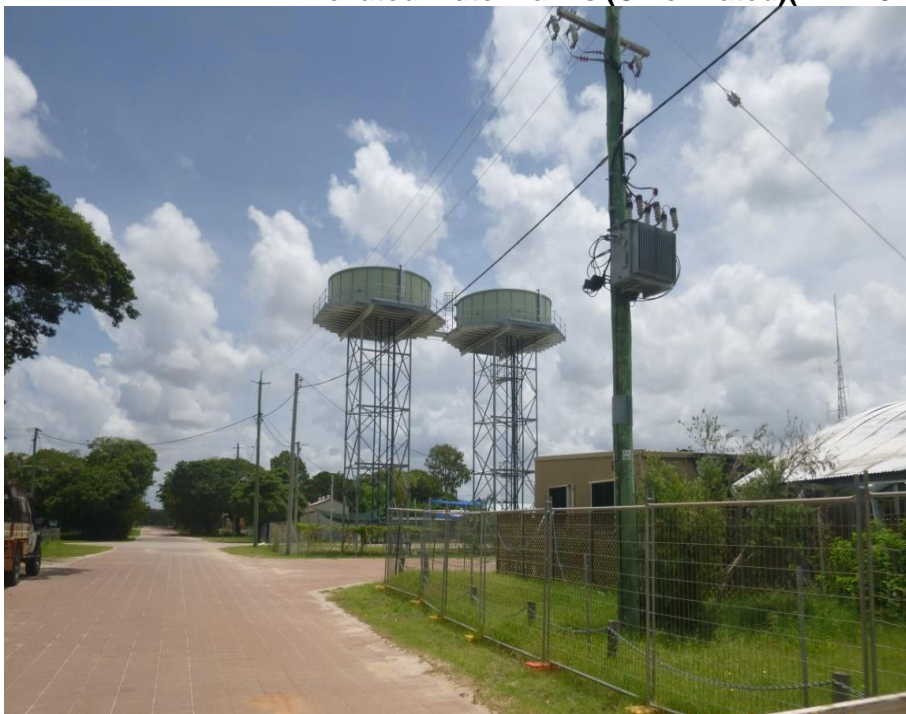
2 Elevated Water Tanks (Chlorinated)(2 x 120KL)
