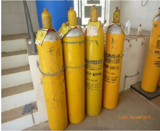
Chlorine Gas Spare Cylinders
