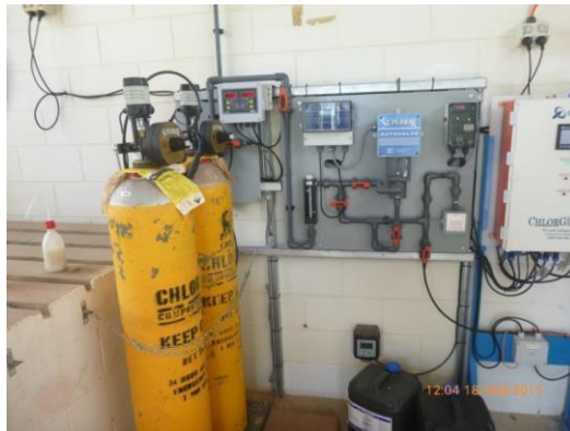
Chlorine Gas System
