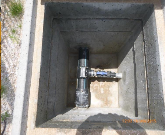
Chlorine Gas Injection Point
