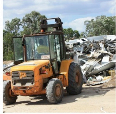
Landfill must deal with very large volumes Pormpuraaw Aboriginal Shire, Sept. 2016
